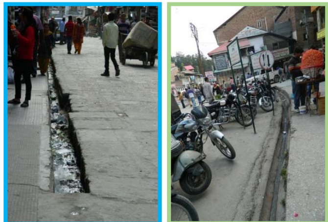
Figure 5: Open drains and trapped solid waste in drains
